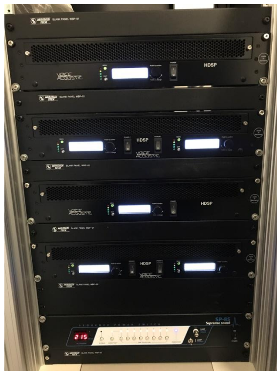
[ Amp Rack _ HDSP-4A,0.4A ]
